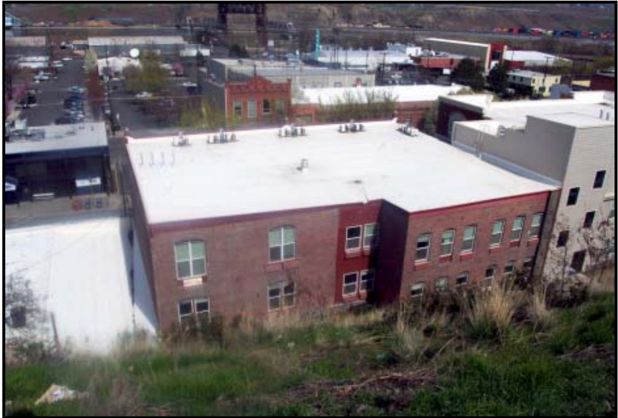
View northerly of the older building from the steep hill to the south.
