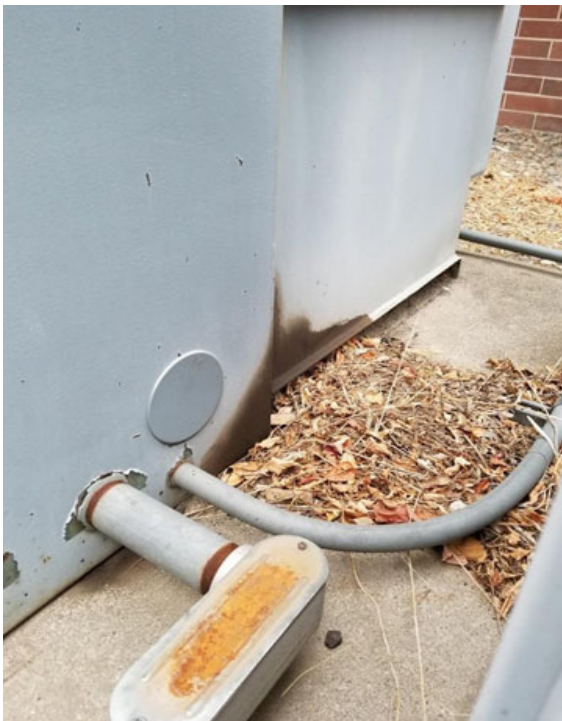
Figure 1. Example of oil leaking from transformer.
