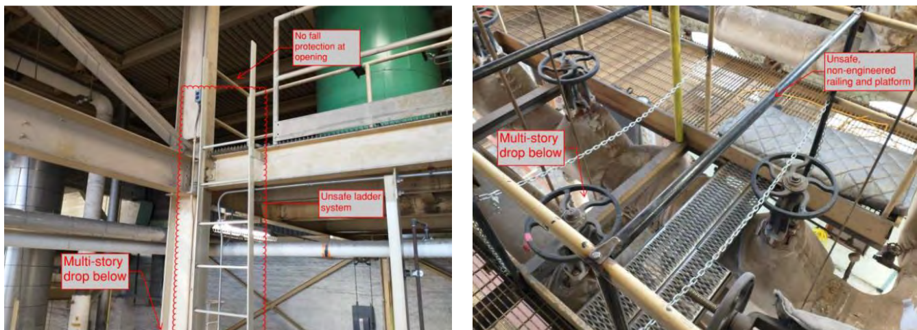
Figure 4. Other examples of unsafe conditions to access critical elements.
