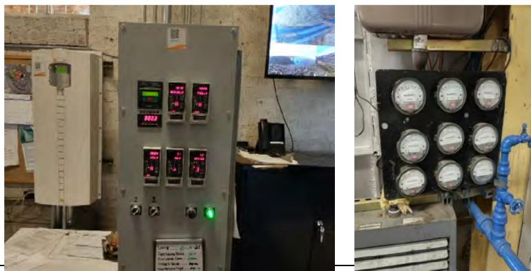
Figure 3. Examples of obsolete gas boiler control and operator station.
