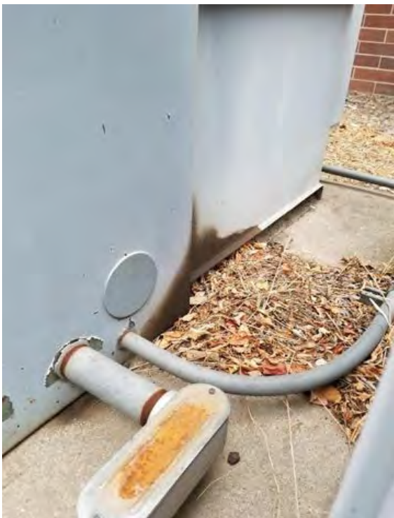
Figure 1. Example of oil leaking from transformer.
