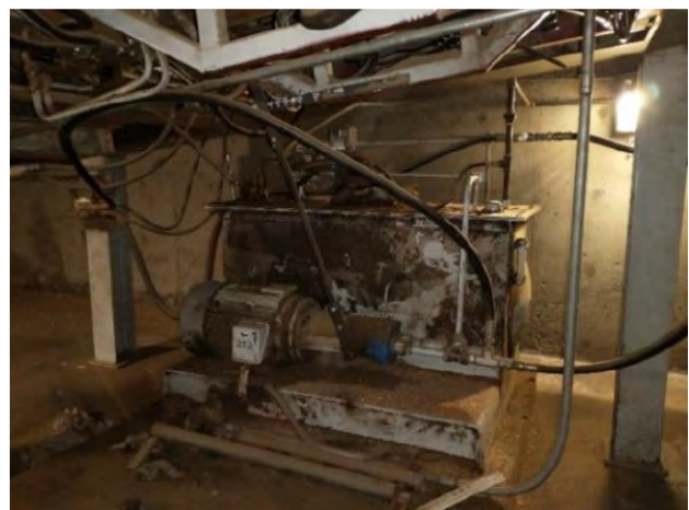
Figure 2. Hydraulic system beyond serviceable life.
