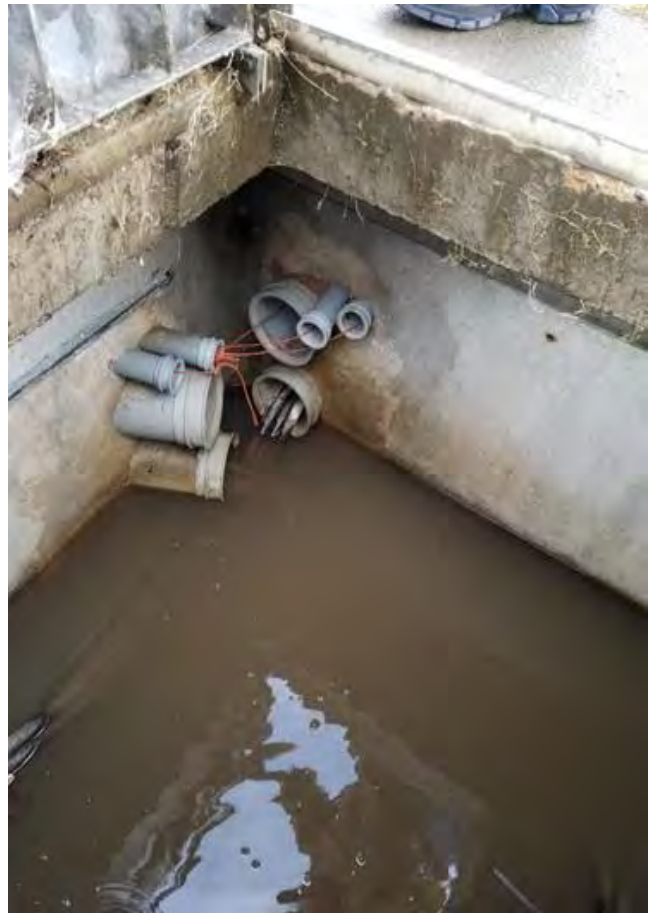
Figure 2. Electrical conduits submerged in vaults.
