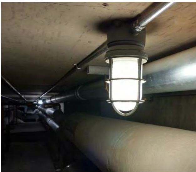
Figure 3. Fluorescent lights still in use.
