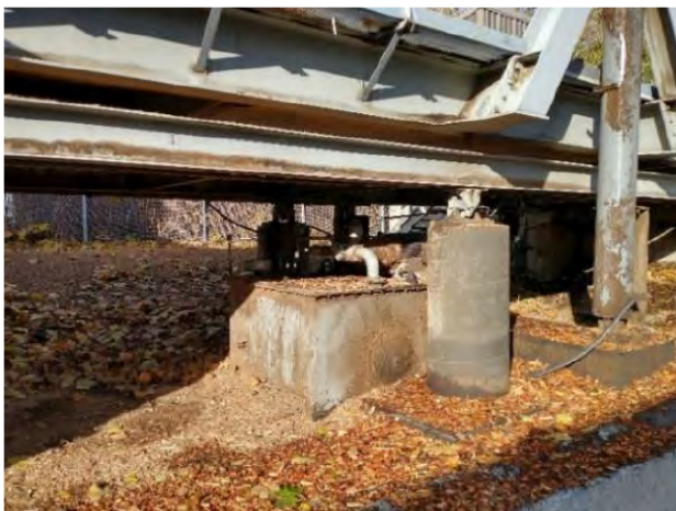
Figure 1. Tipper hydraulics in poor condition surrounded by combustible materials.
