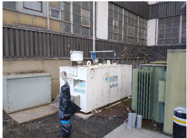
Figure 2. Existing fuel tank.
