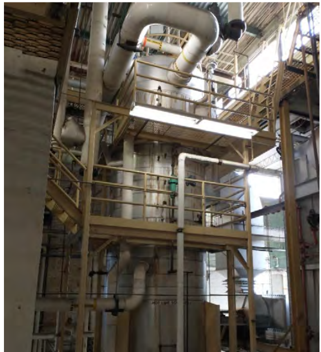
Figure 2. Hot Lime Softener #2.
