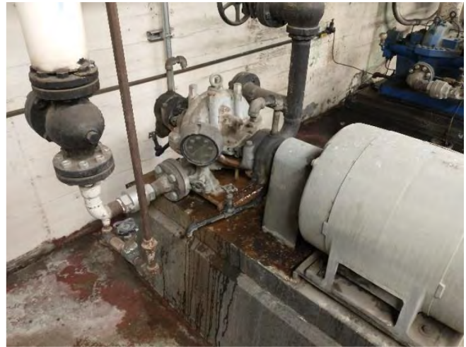
Figure 2. 64-year-old feedwater pump showing heavy leakage.
