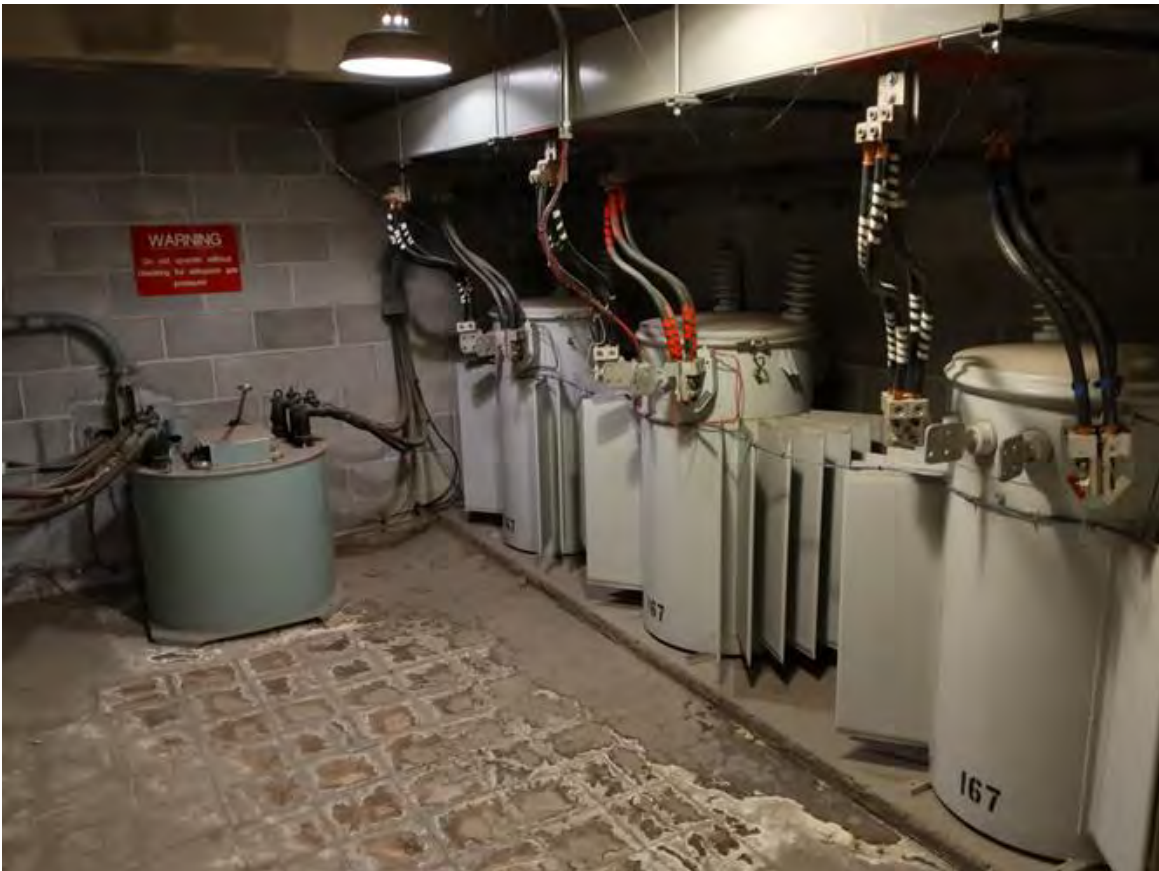
Figure 1. Aged transformer and electrical equipment in Admin south basement.
