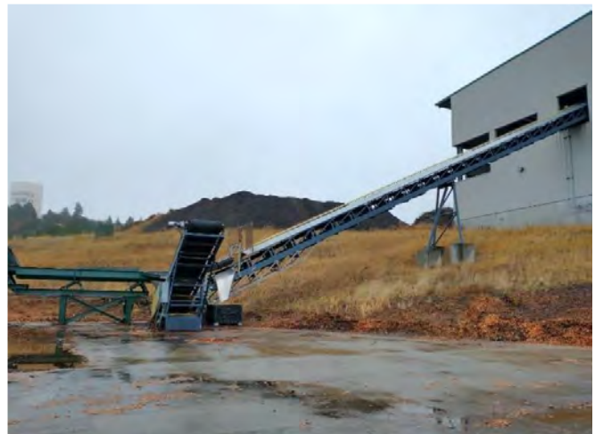
Figure 2. Wood chip conveyance system.
