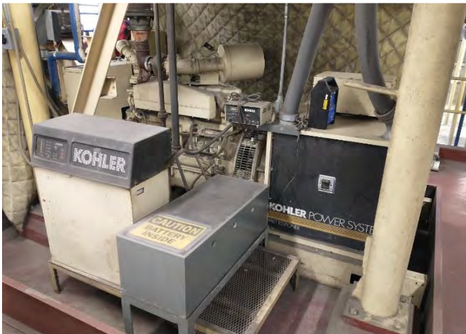
Figure 1. Aged generator at the Energy Plant.
