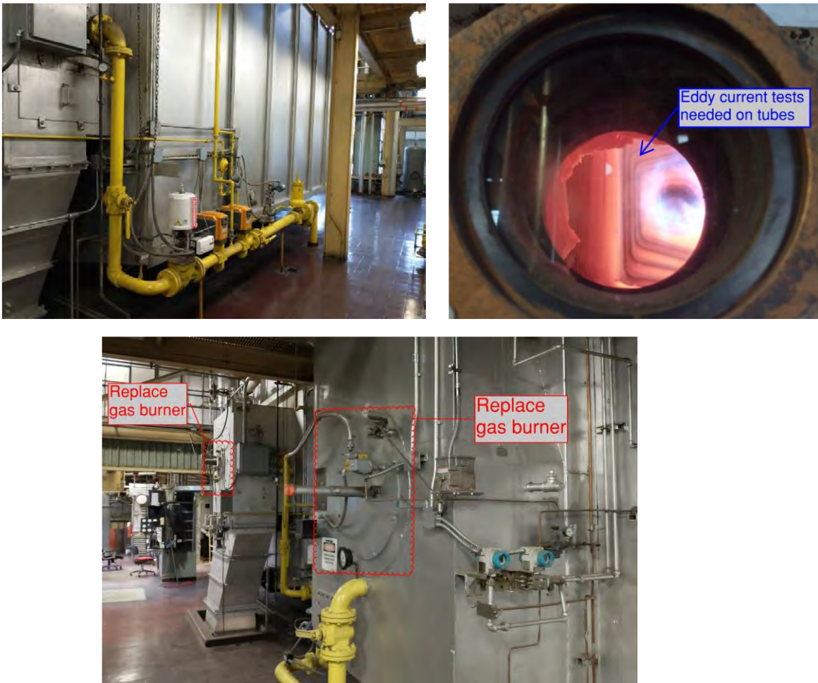
Figure 1. Detailed views of the natural gas boilers.
