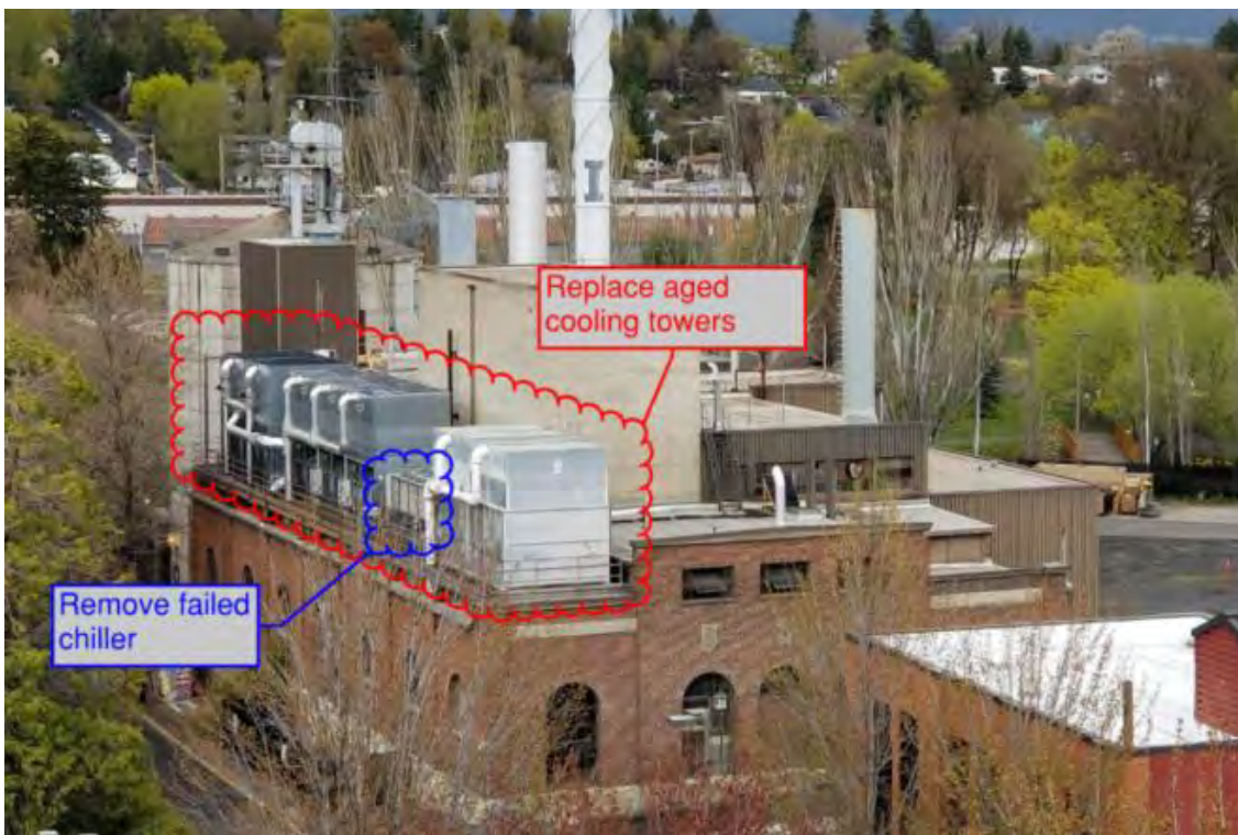
Figure 1. Cooling towers at NCCP
