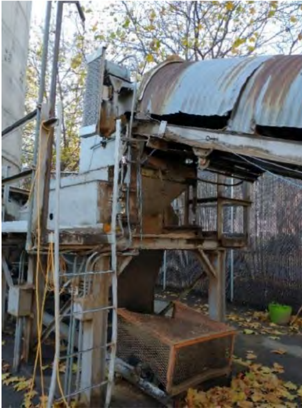
Figure 3. Aged wood conveyance system in poor condition.
