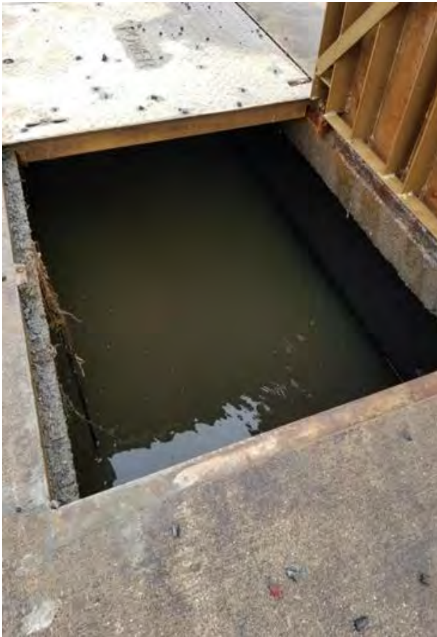
Figure 1. An electric vault that is completely submerged. Condition of equipment is unknown.
