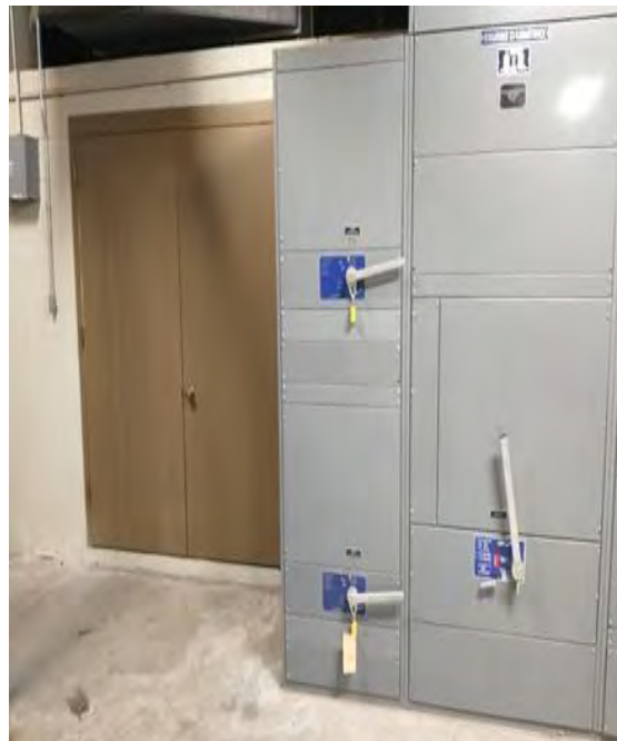
Figure 2. Conditions in transformer room dangerous enough to require Arc flash PPE before entering.
