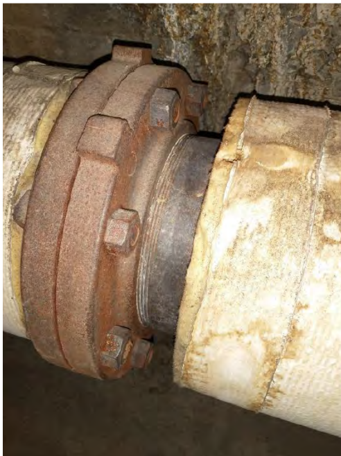
Figure 1. 95-year-old threaded pipe poses a safety hazard.
