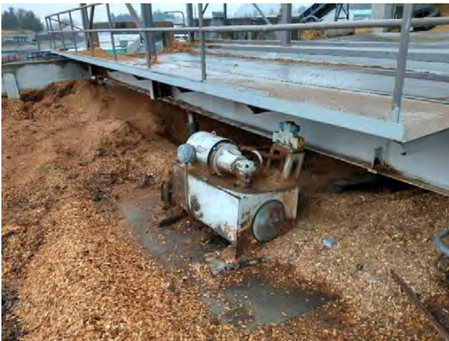
Figure 1. Tipper hydraulics surrounded by flammable material.
