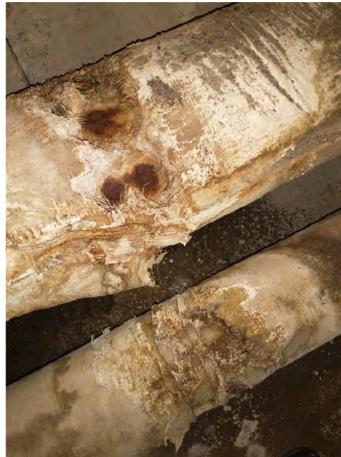
Figure 2. 95-year-old threaded pipe is rusting through.
