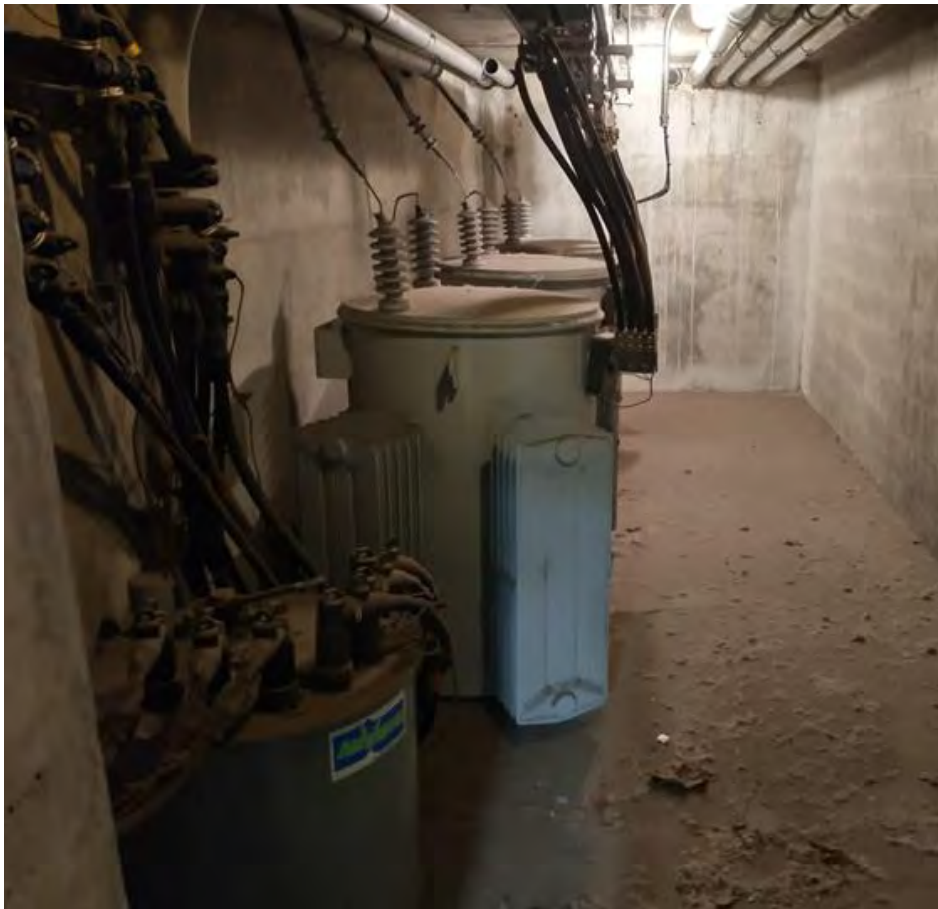
Figure 1. Aged transformers and electrical equipment in CNR basement.
