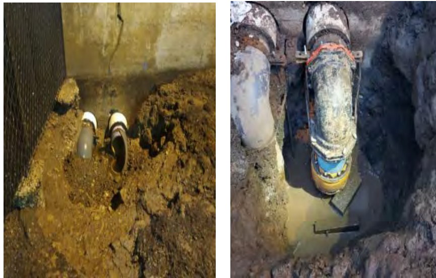
Figure 1. Joint that failed at NCCP in January 2021 and flanged joint installed after failure.
