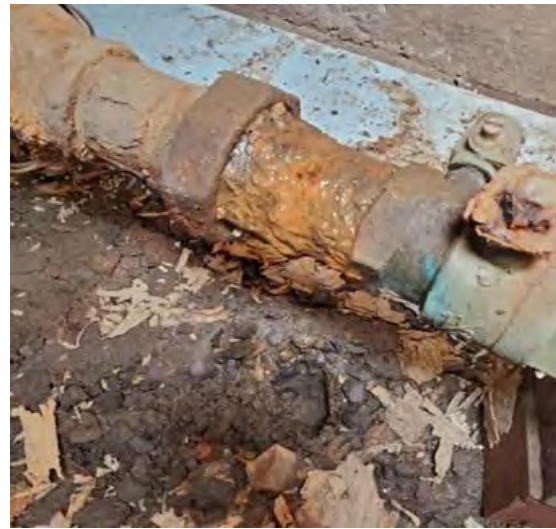
Figure 2. Leaking water line in vault.
