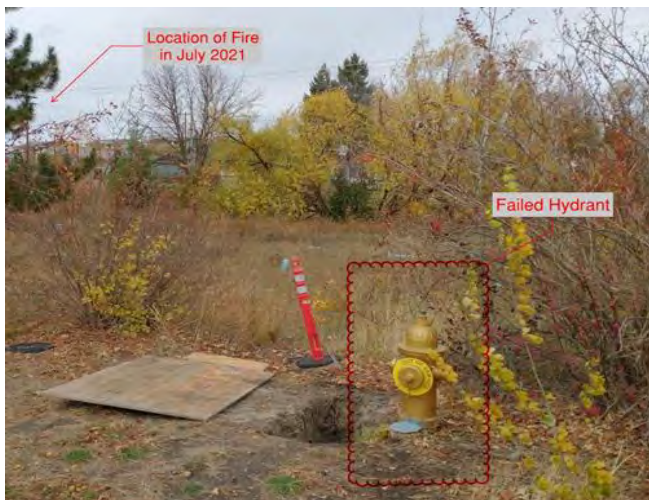
Figure 2. Failed hydrant on campus near a brush fire in July 2021.
