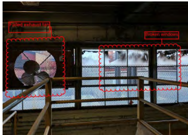
Figure 2. Failed exhaust fan and broken windows.
