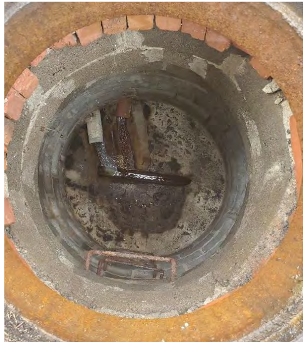
Figure 1. Bricks falling out at a damaged manhole.
