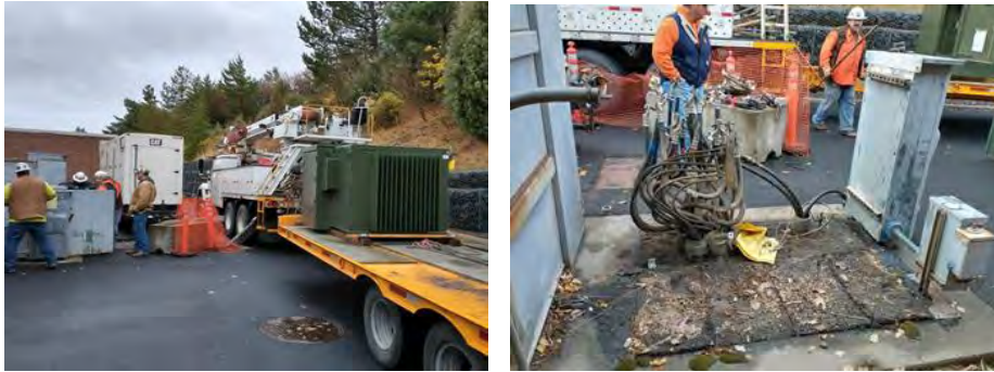
Figure 1. Portable generator in place while transformer is being removed/replaced.
