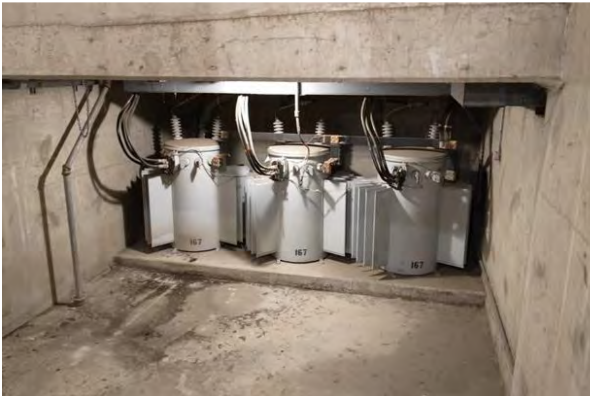
Figure 1. Aging transformers in PEB basement.
