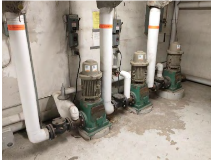
Figure 1. Aged condensate pumps in hot well room.
