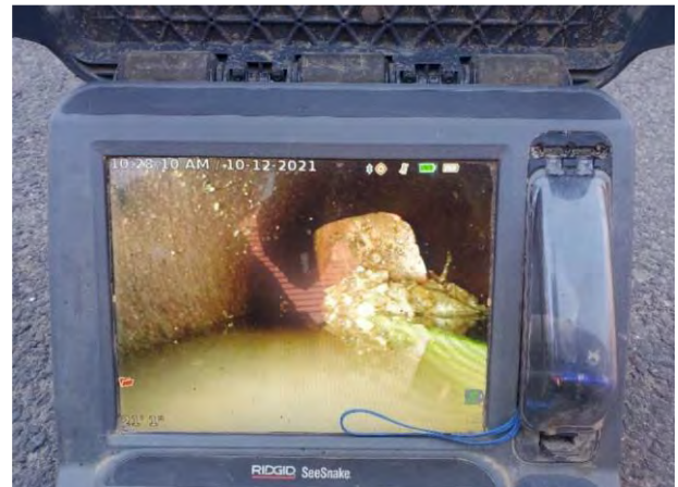
Figure 1. Broken section of pipe in Janssen Engineering service line.
