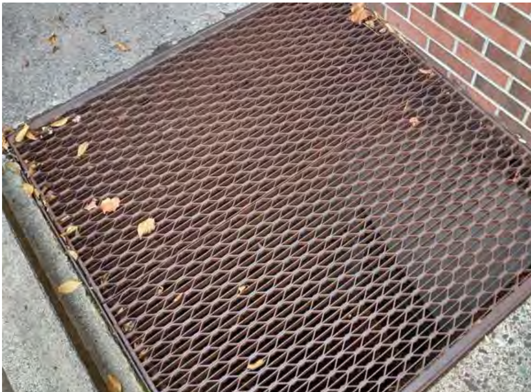
Figure 1. Poor, unsafe access to Art & Architecture north transformer room.
