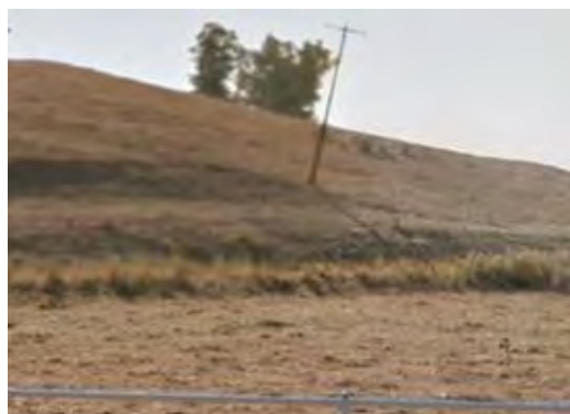
Figure 2. Pole leaning, risking line slap and downed lines.
