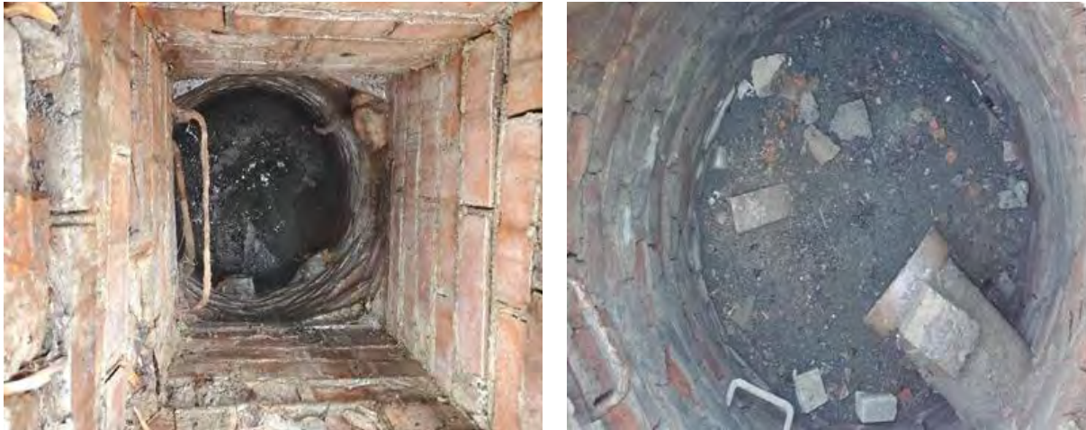
Figure 1. Poor condition brick manhole by ISUB (left) and by Morrill Hall (right).
