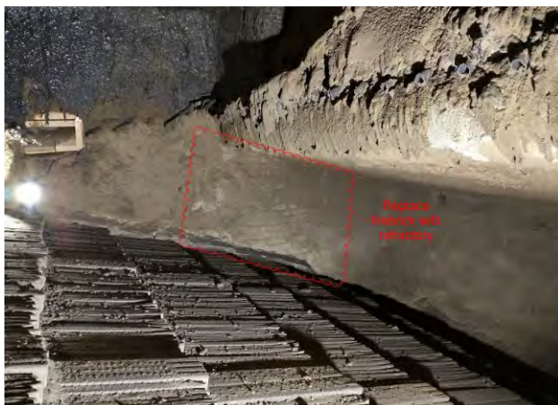
Figure 2. Exposed firebrick in boiler.
