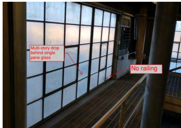
Figure 3. Severe fall hazard behind window.
