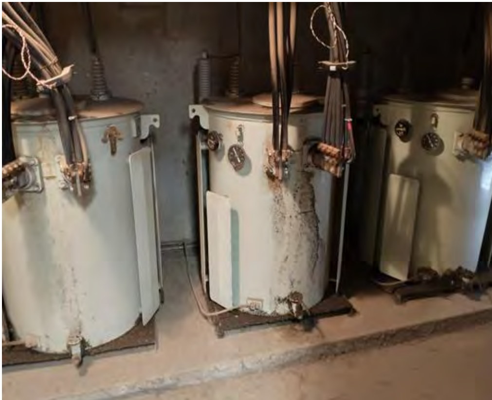
Figure 1. Existing pot transformers in Hartung.
