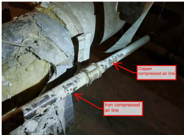
Figure 1. Iron compressed air lines.
