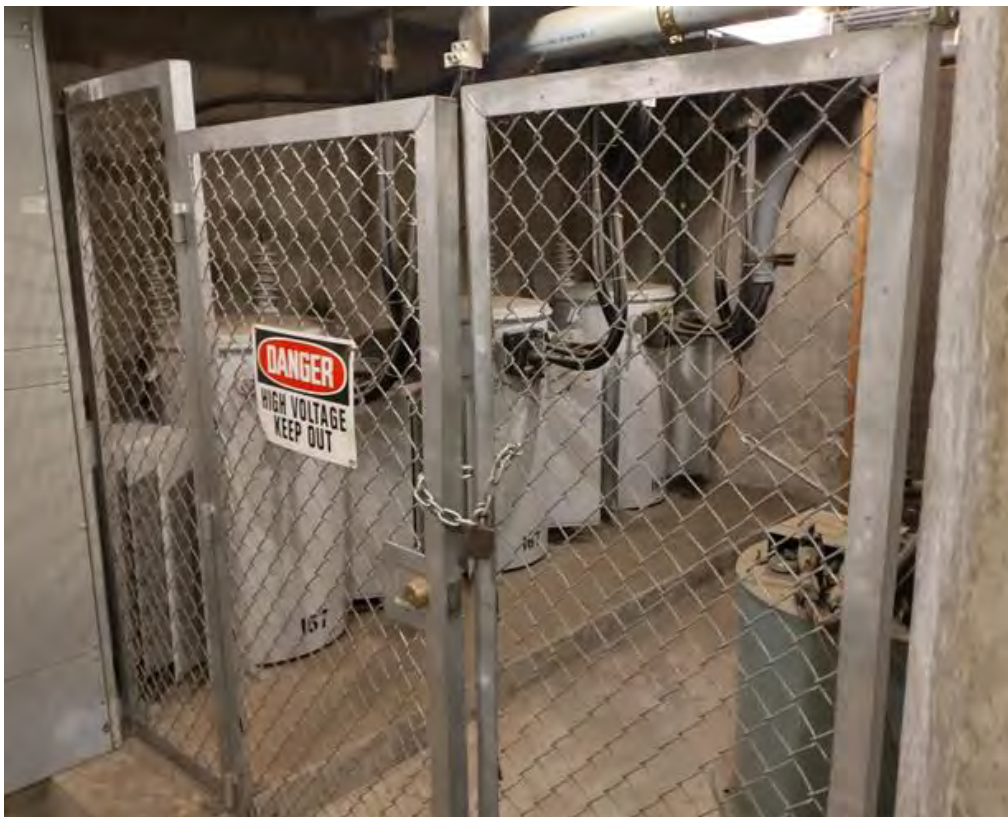
Figure 1. Unsafe, aging transformers and electrical equipment below the swimming pool.
