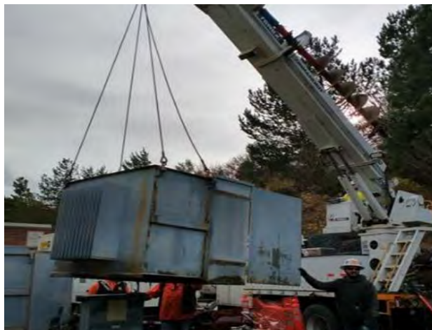
Figure 2. The replacement of transformer can take months.
