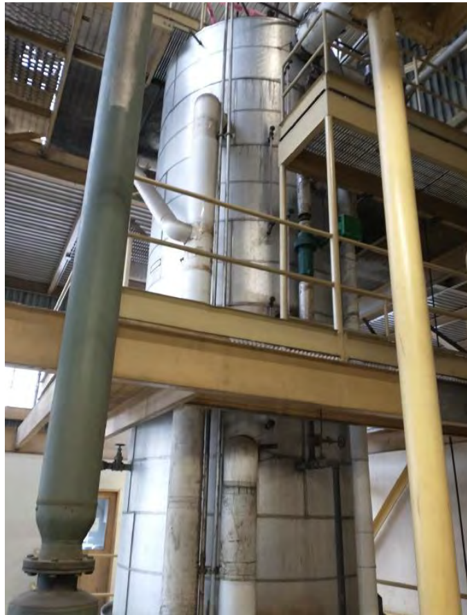
Figure 1. Aged Hot Lime Softener #1.
