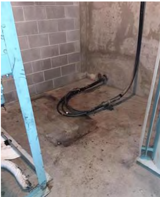
Figure 1. Unsafe conductor splice laying on the floor after emergency repairs in 2019.
