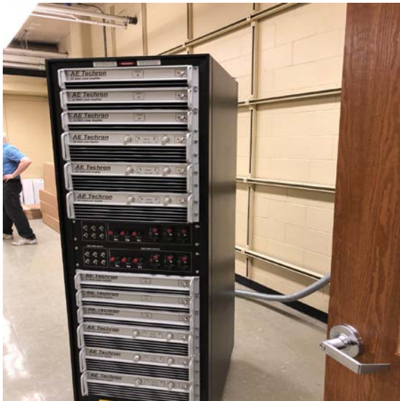
Figure 3: Amplifiers moved and installed in the new space.
