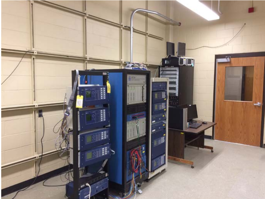
Figure 5: RTDS, some of the test equipment racks and power amplifiers in remodeled lab space
