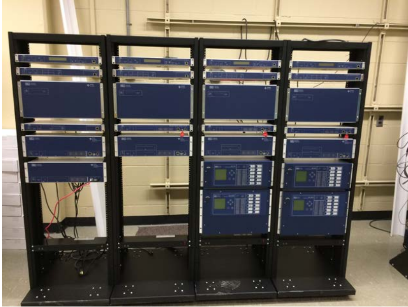
Figure 6: Some of the test equipment for the expanded power lab along with new equipment racks
