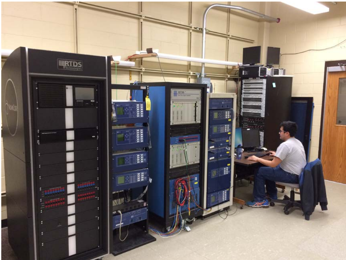
Figure 7: Testbed with the addition of the new RTDS NovaCor rack.
