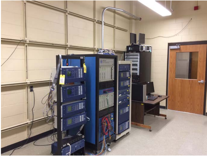
Figure 5: RTDS, some of the test equipment racks and power amplifiers in remodeled lab space
