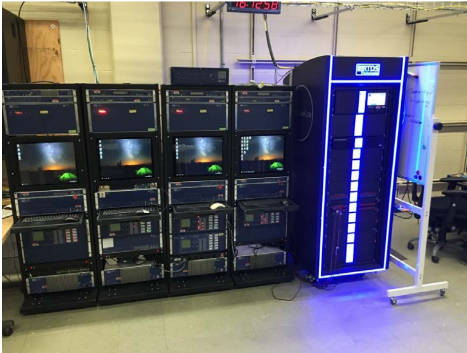
Figure 5: Completed and Operational PowerLab Components of the ISAAC Testbed. Four SEL power control equipment racks (left) and new RTDS NovaCor (right). Each SEL equipment rack contains equipment roughly equivalent to a power substation.
