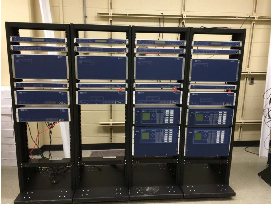
Figure 3: Some of the test equipment for the expanded PowerLab along with new equipment racks (each rack will simulate a complete power substation's control).
