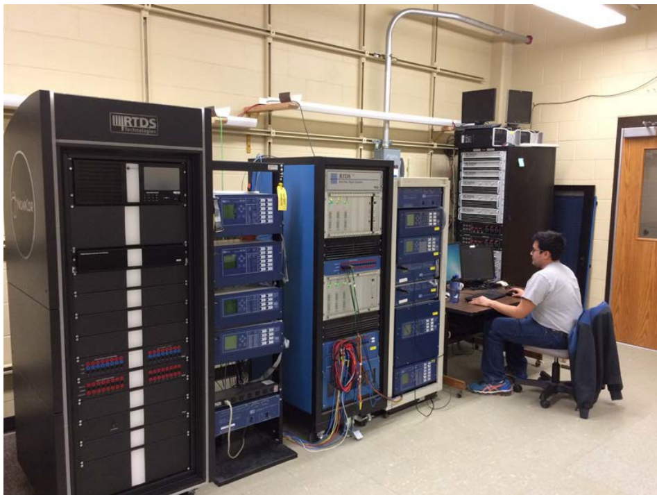
Figure 4: PowerLab Component of the ICS Testbed with the addition of the new RTDS NovaCor rack (to the left).
