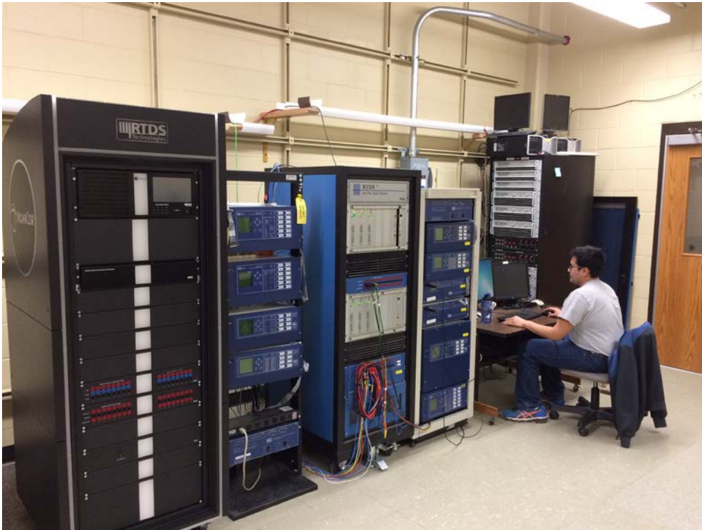
Figure 7: PowerLab Component of the ICS Testbed with the addition of the new RTDS NovaCor rack (to the left).
