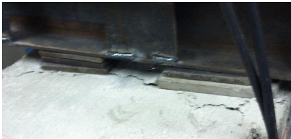
a: Bending Failure – Concrete Crushing
