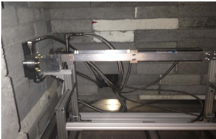
Figure 1 Water cooled target system inside the shielded activation area.
