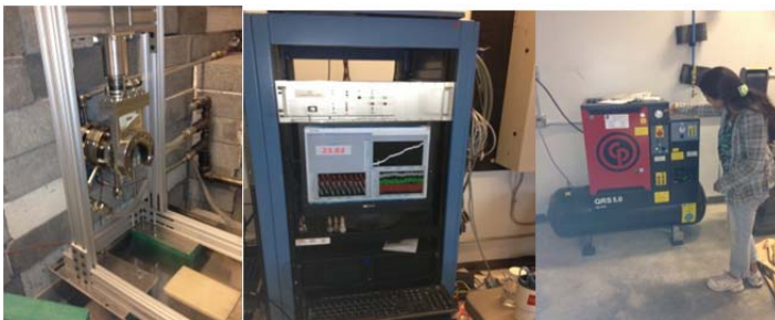
Figure 8 - the picture on the left is the target and converter on the end of the accelerator. The converter is water cooled, the target is air cooled currently, but, will switch to water cooling for production. The center picture is the control system developed to monitor energy during production and temperature of the target. The right picture is the high capacity compressor.
