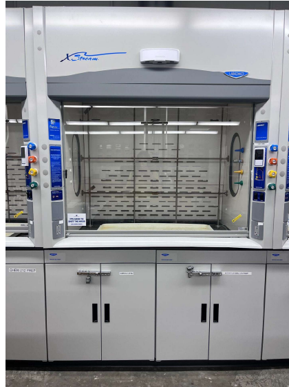
Photo above: Modern fume hood in the Science Building
