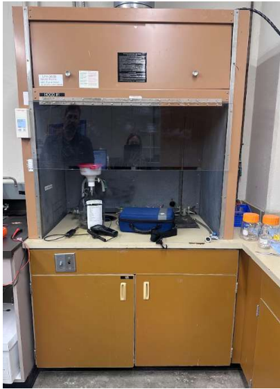
Photo above: Aging fume hood in the Science Building
